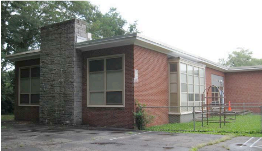
4. North view of north kindergarten wing and play yard, camera facing southeast.
