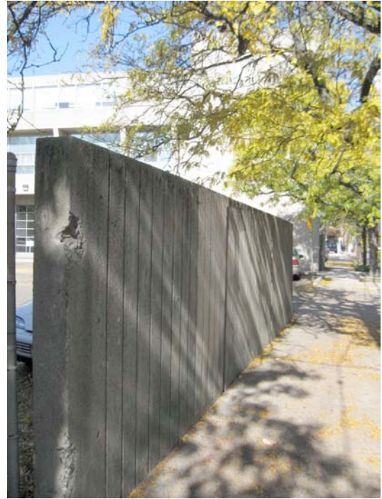
9. Southeast perimeter wall - screening parking area from pedestrian walk — continuation of concrete vocabulary.
