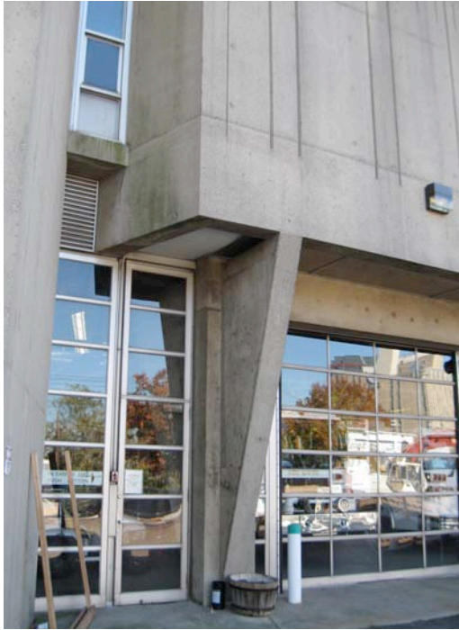
8. North Elevation Door details showing how doors as functional openings are suppressed in favor of the sculptural treatment as glazed infill between solid masses,.
