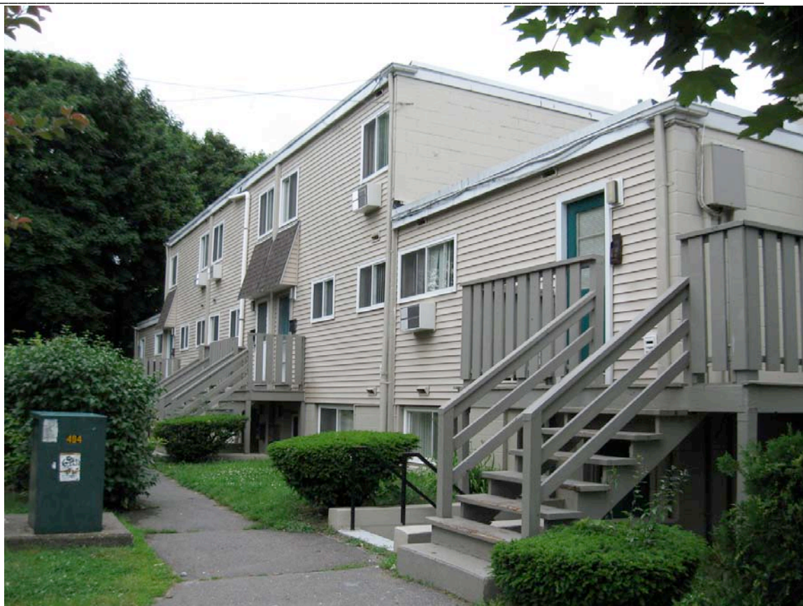
3. Entry side of Duplex-over-flat building type; camera facing southwest from Goffe Street.
