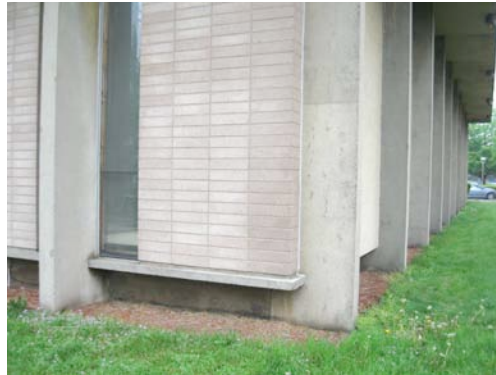
7. Construction detail showing “floating” floor slab, concrete piers, vertical slot glazing, and non-structural 4” block infill.
