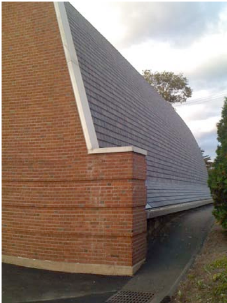
5. View – detail of façade and roof at southeast corner, camera facing north
