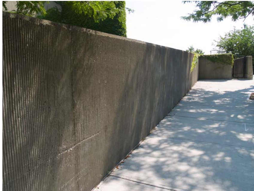
Photo 9. South detail view of the perimeter wall, camera facing east. The finish of exposed concrete is a narrow ribbed texture which gives the building a surprising refinement, contrasting with the hardness of the material.
