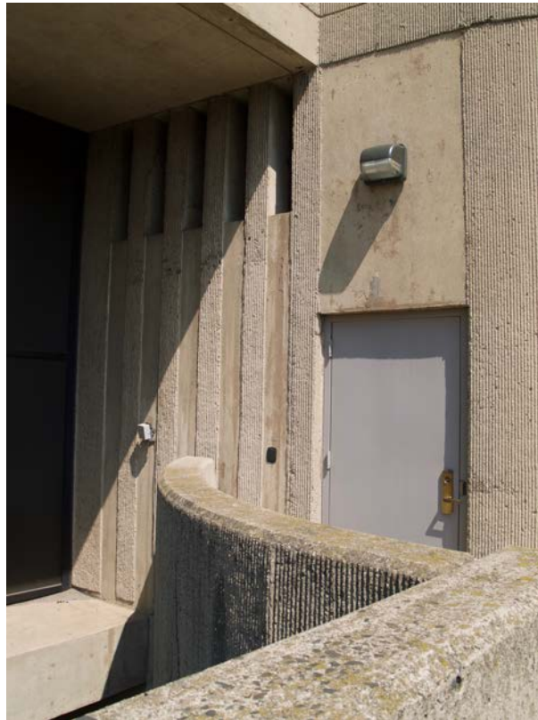
Photo 11. South view of east stair exit to State St. North, camera facing northwest, showing concrete details.
