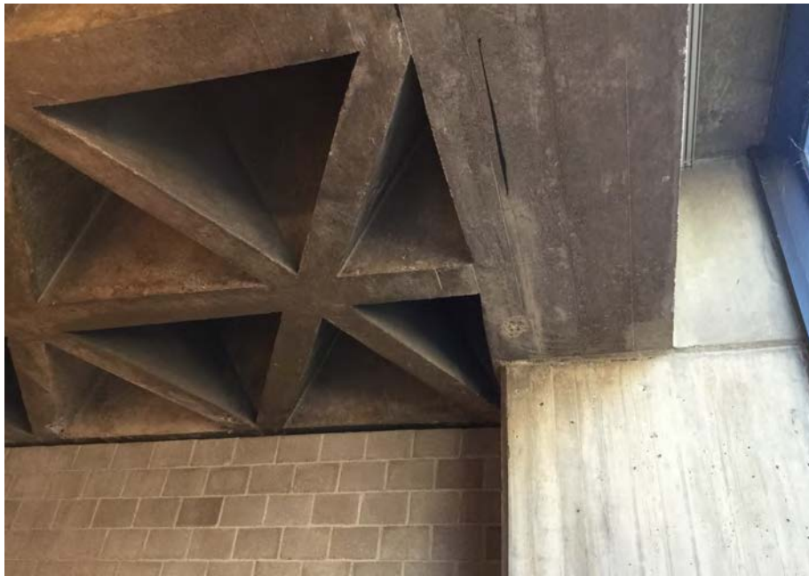
Photo 12. Interior view of Louis Kahn Building at Basement level west wall showing floor/ceiling construction, concrete frame, interior wall finish of concrete masonry bricks, and curtain wall glazing; camera facing south. Note how the structure is held back behind the glass curtain wall.
