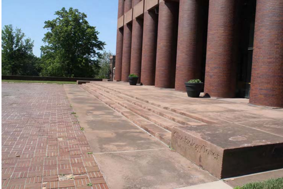
Photo 14. East view of Kline Biology Tower plaza with the base of the tower; camera facing south.
