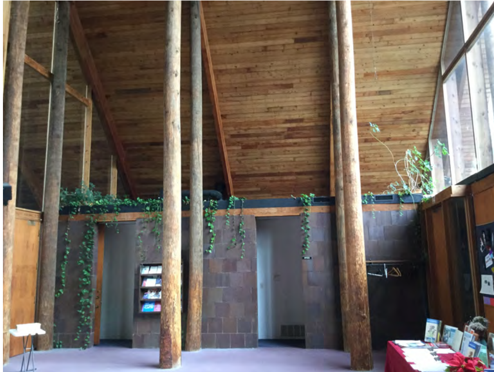
Photo 12. Interior view of the Copeland Room, camera facing south. Doorway at rear leads to pastor's office (right) and Sunday school rooms (left) along the south side.
