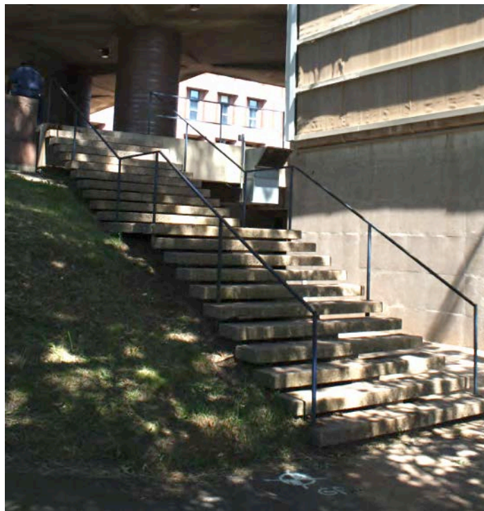
Photo 9. South view of the building end wall; camera facing west. Note the open riser stair cantilevered on a central line of support.
