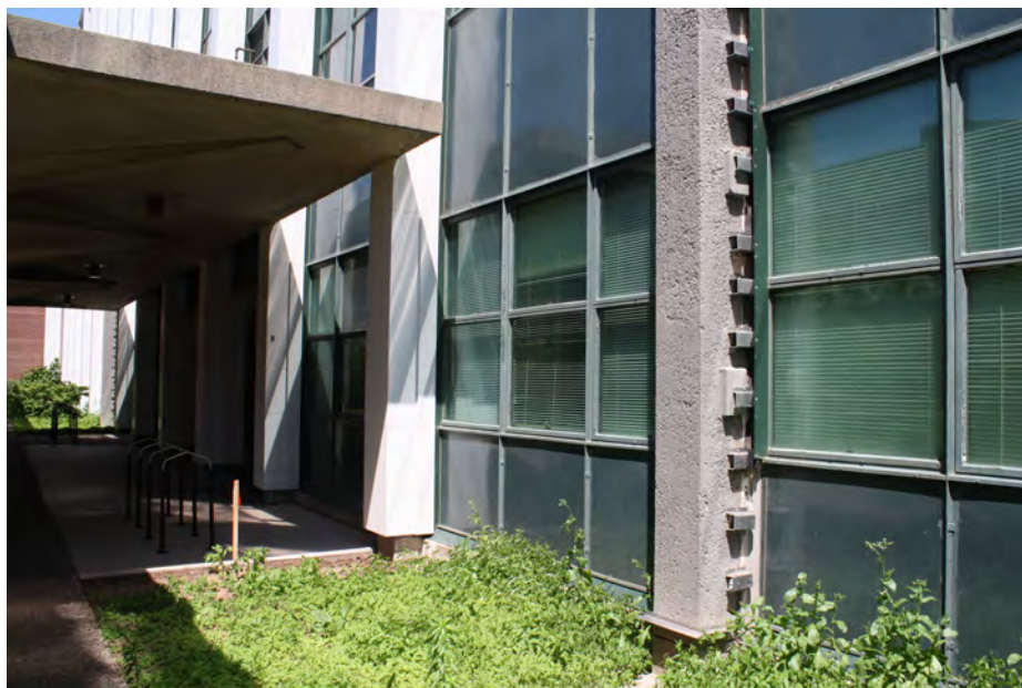
Photo 7. Detail view of the west side at the plaza level; camera facing northeast. Exploratory demolition has exposed the concrete column construction.
