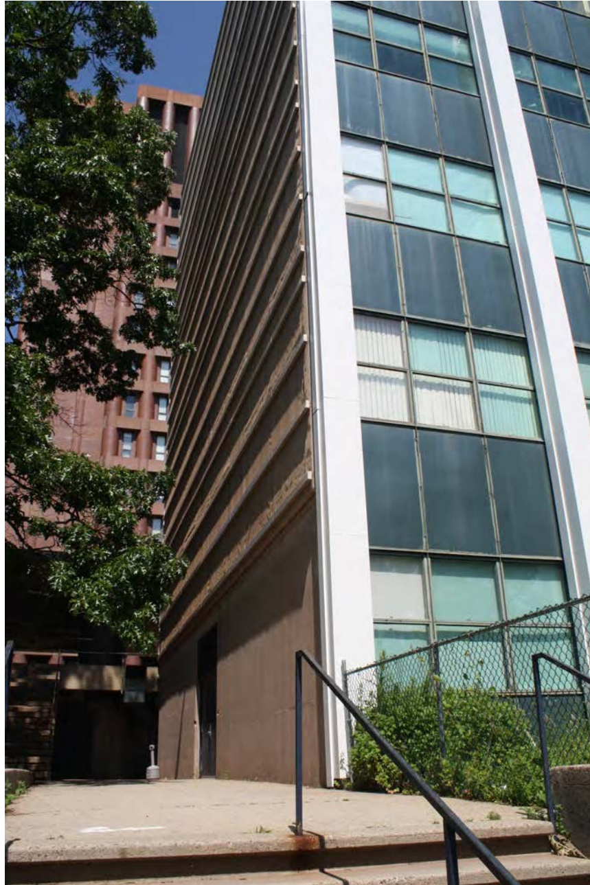
Photo 10. Southeast view of the building end wall; camera facing west. The original marble veneer cladding on the north and south end walls has been removed.
