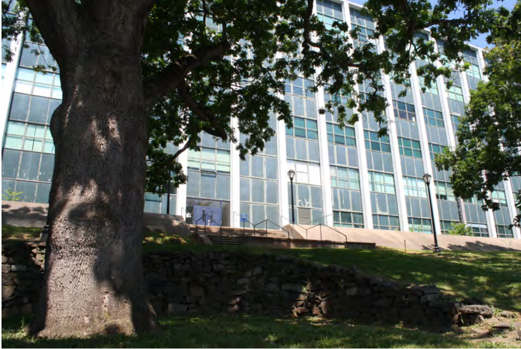
Photo 6. Detail view of the east side showing the first level entry doors and typical curtain wall; camera facing west.
