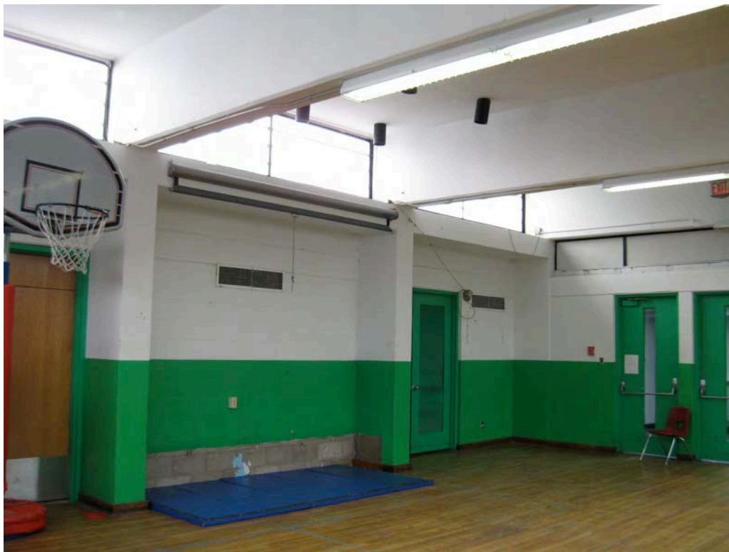
Photo 8. Interior view of the Multi-purpose Room; camera facing southeast. Note structural system of piers supporting concrete girders with clerestory windows.
