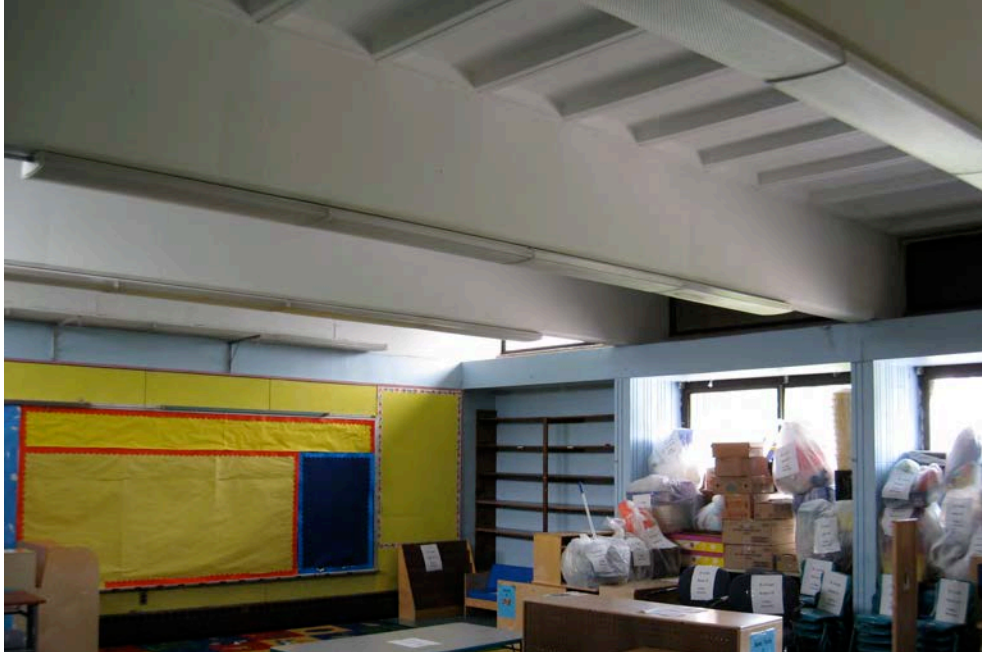
Photo 11. Interior view of typical classroom north wall; camera facing north. Note (blocked by boxes) the full-length windows open to an outdoor courtyard for each classroom.
