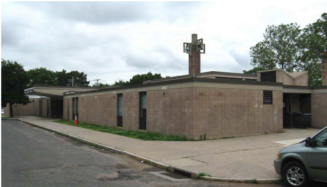
Photo 4. South view of Helene Grant School, camera facing north. The entrance canopy is at left.
