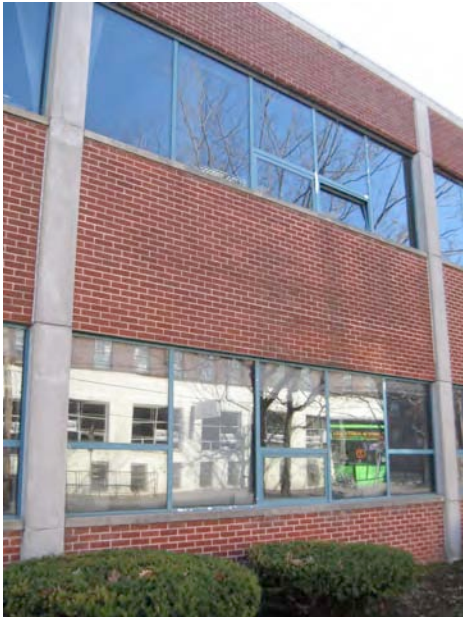
2. N view from Chapel Street, camera facing south showing unaltered portion of façade.
